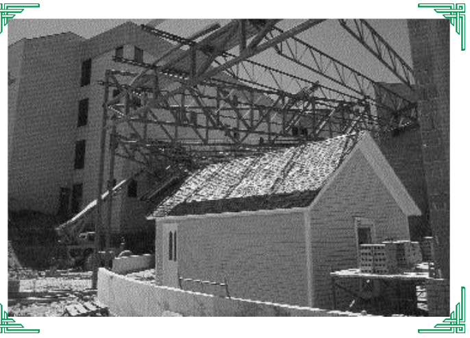
The original ASO building and Cabin were placed in their new sites during the early stages of the construction of Heritage Hall, October 1993. [Kirksville magazine, Spring 1994]
