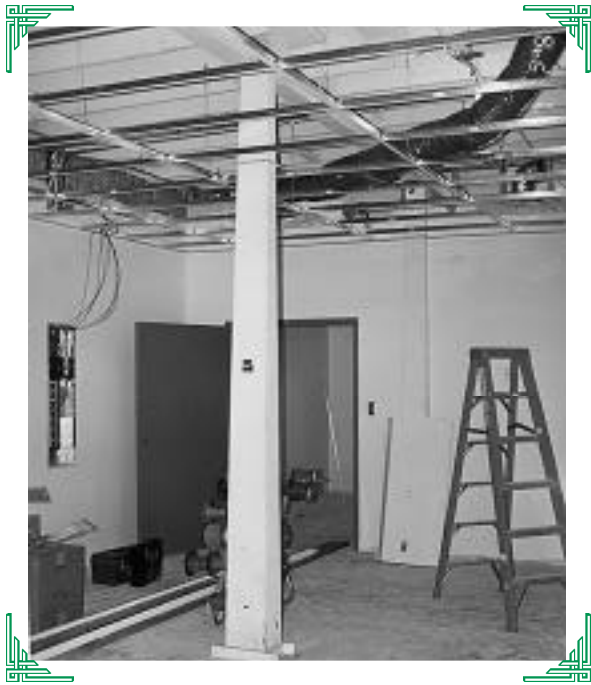
Construction of the “overflow” artifact storage area and exhibit workshop at the Annex Building, September 1998. [Museum Archives]
