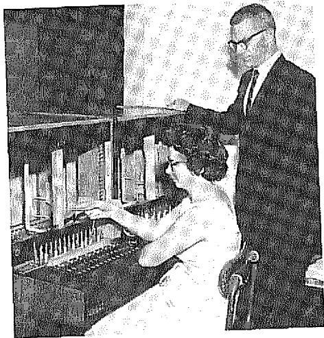
Mr. Clare Pearson, KOH Administrator, looks on as Mrs. Christine Sudemeyer operates the new switchboard, installed 1963
