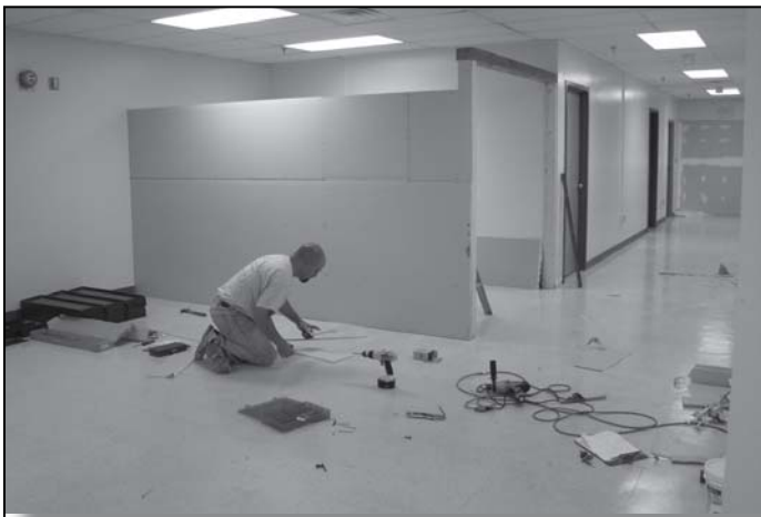
Rob Clement, Exhibit Preparator, constructs new office space for ICOH staff from space, which formerly housed the Osteopathic Theory and Methods
